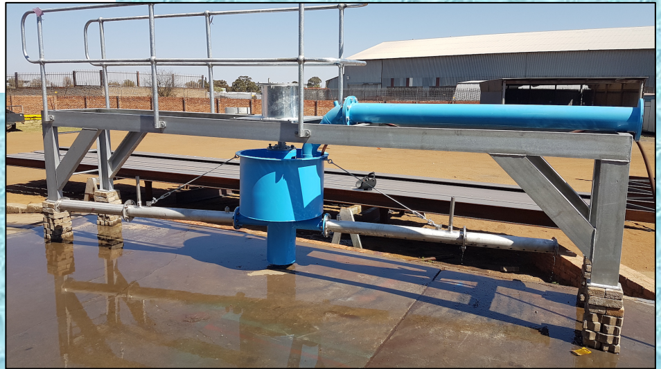
Aquelle 0-11 l/s biofilter
